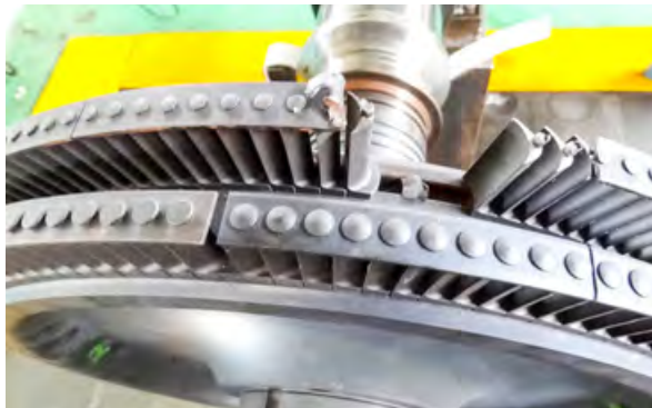
Broken blades / buckets.
