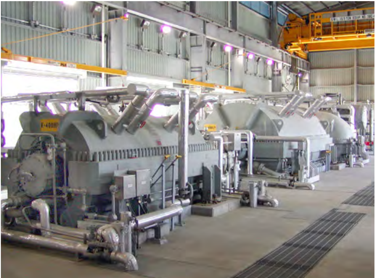
Crack gas train – Elliott 2SNV9 steam turbine driver with 88M61 and 60M61 compressors.
