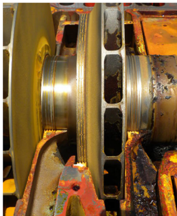
Figure 1. Corrosion on a chlorine compressor.
