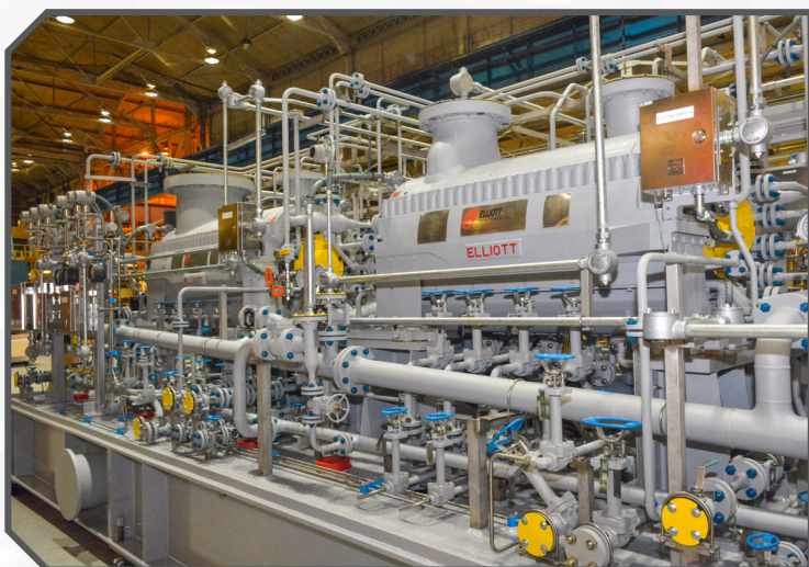
Elliott Group: End flash gas compressor package.
