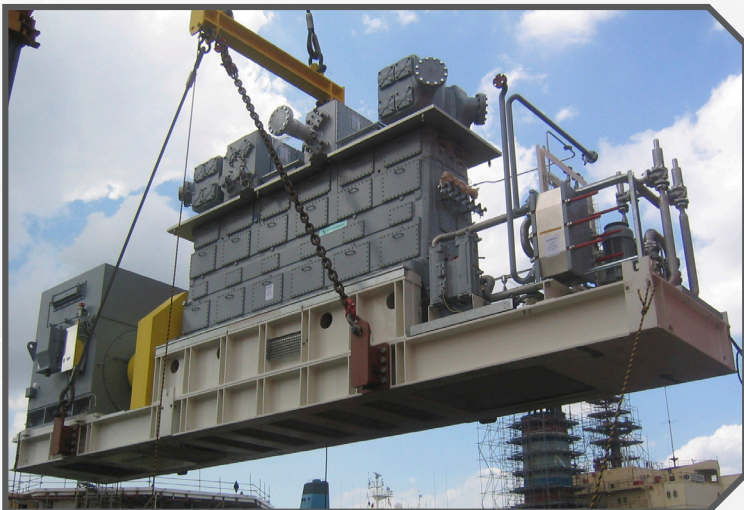
Burckhardt Compression: Laby-GI compressor being transferred to a ship for onboard installation.
