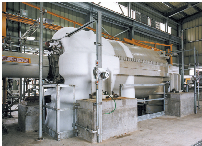
Figure 4. Propylene refrigeration compressor.
