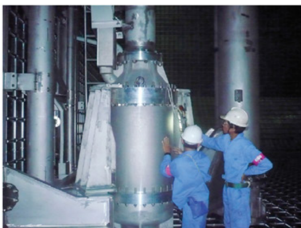
Figure 1. A submerged motor cargo pump inside an LNG carrier.
