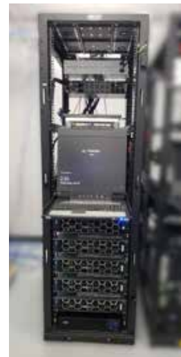
Mitsubishi Power’s Netmation Protect Pack provides cybersecurity for turbine control systems to the NERC CIP requirements.
