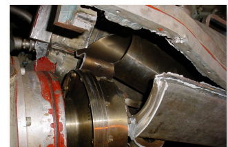
Damaged coupling spacer and coupling guard.
