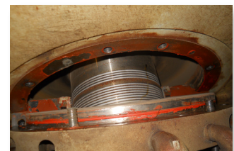
Damaged seal housing.
