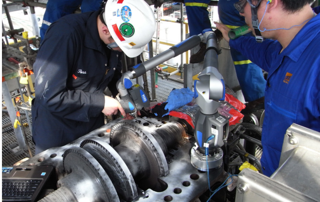
Elliott engineers on the turbine deck at the refinery, measuring rotor dimensions with a portable CMM and hand-held laser scanner.
